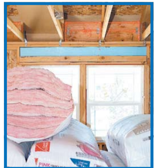
Raised heel rafter trusses allow for insulation to be installed across the entire attic for improved energy efficiency in the ReStore home.
