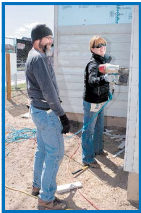
Volunteer Bruce Schroeder and ReStore director Sophie Paez work with one another to install siding on the Bend Area Habitat for Humanity ReStore home.
