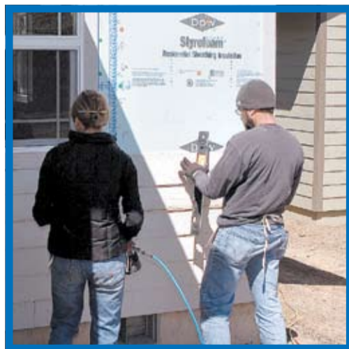
Half-inch Styrofoam sheathing, donated by Dow Chemical, adds additional wall insulation and protection from water vapor condensation in the wall cavity of the ReStore home.
